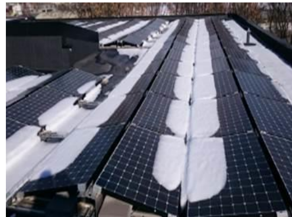
Figure 7: Example of non-integrated, traditional photovoltaic panels placed without regard for snow removal on the roof of Block 4 of Powerhouse Kjørbo (Norway) (Ødegården, 2016).
