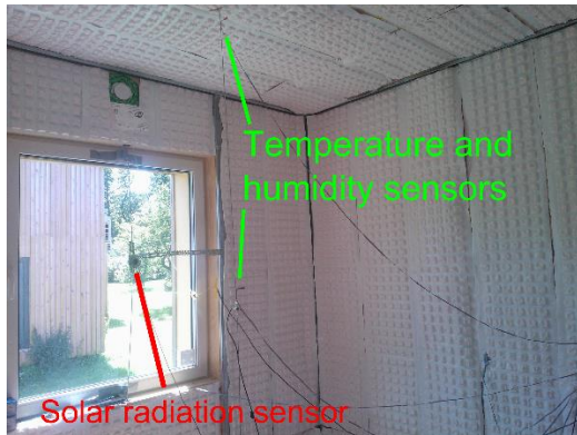
Fig.4. Location of solar sensors at the window, temperature and humidity sensors on vertical line and PCM on the walls and ceiling.
