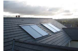
Flat plate collector, Ireland
