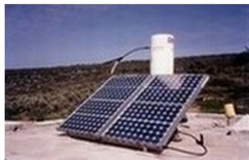
Multi Solar System, MSS Millenium Electric, Israel
